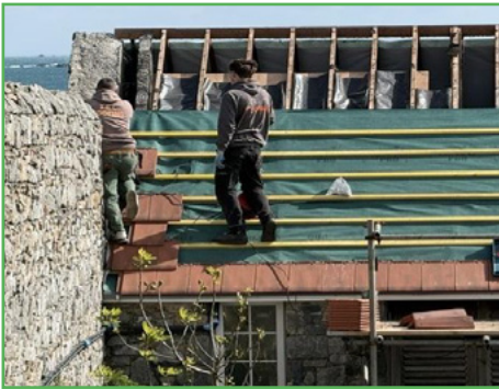
Lihou House roof after the Storm Gorette
